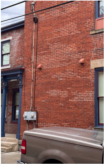
Example of a meter and vents placed on secondary facade.
