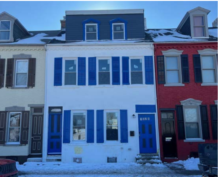
Example of an inappropriate dormer addition, which removed an original dormer and introduced non-historic proportions.
