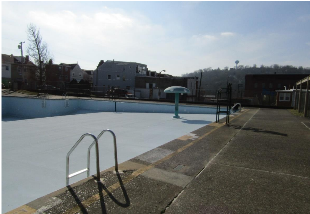
Figure 3.b-5: Pool deck discoloration indicates a need for cleaning.
