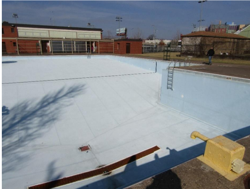
Figure 3.b-1: Pool access does meet current standards.
