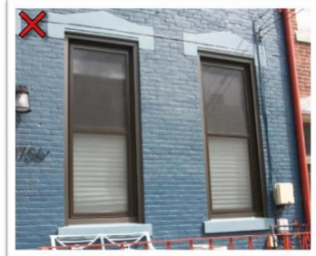
These aluminum replacement windows do not fit well in the existing openings. Further, the metal gives an industrial feeling that is not appropriate to the house.
