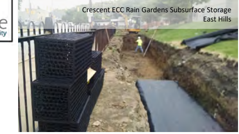
Subsurface Storage Chambers
