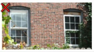
These replacement windows do not fit within the existing openings and are the wrong shape. The false muntin grid is not appropriate for the building, and the bright white vinyl sash provides too much contrast.
