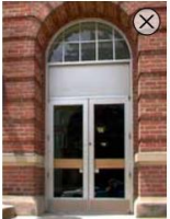
Avoid installing a new door that is out of character with the building.
