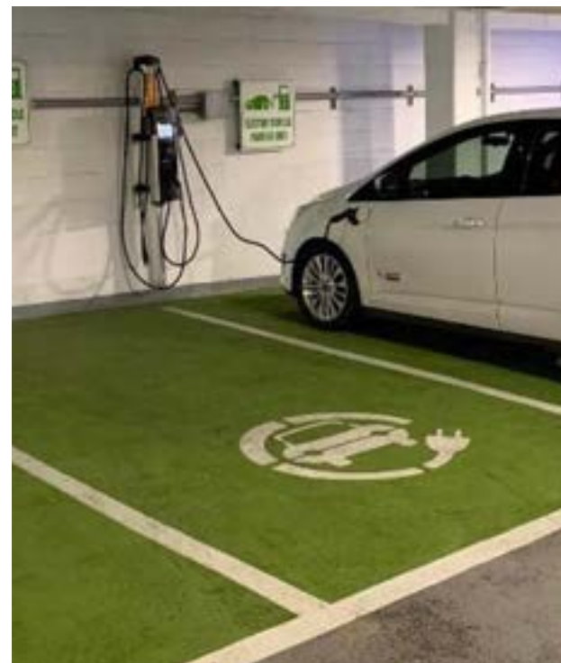
An example of EV infrastructure in a publicly accessible parking garage
