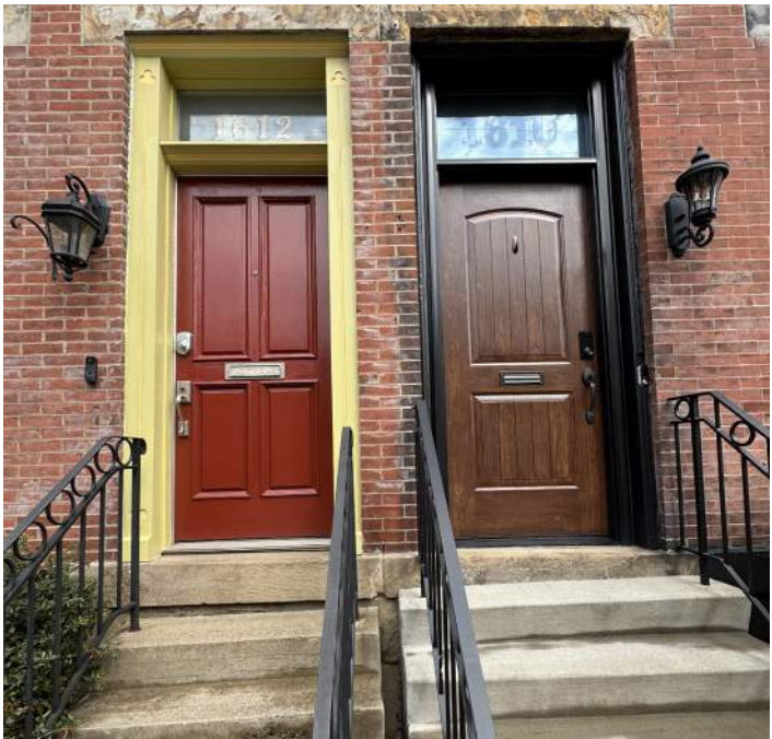
Appropriate replacement door (on right) is in keeping with the character of historic doors.
