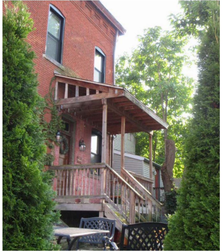
Appropriate new porch on non contributing facade.
