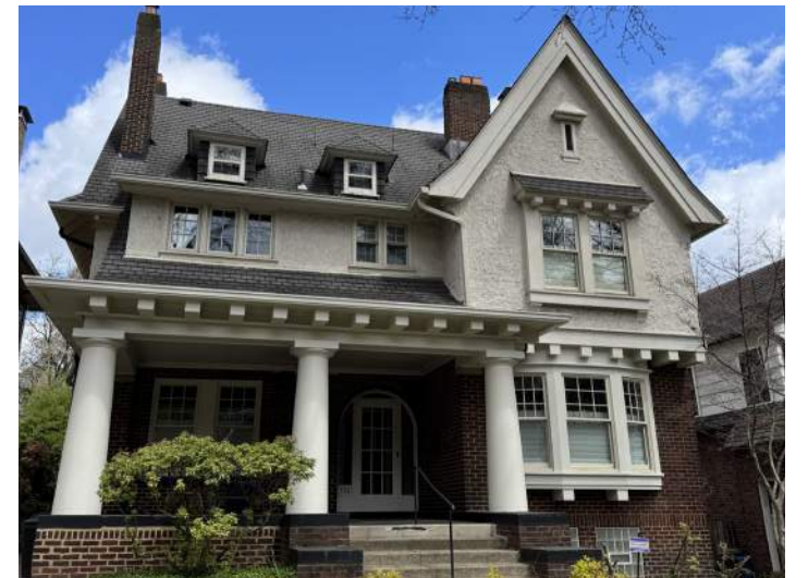
Stucco should be maintained and repaired to keep a consistent appearance, color, and texture.
