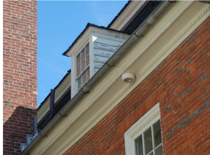
Modern facade lighting is concealed under the eave and the fixture color blends in; this is an appropriate installation.
