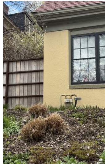
Example of a meter located on a primary facade.
