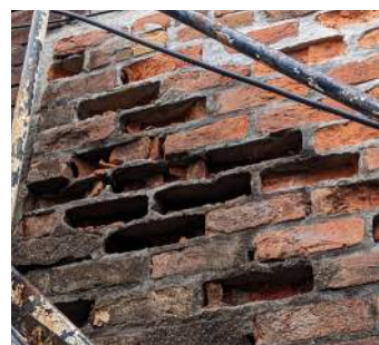
Example of deterioration to masonry caused by inappropriate strength mortar repair.
