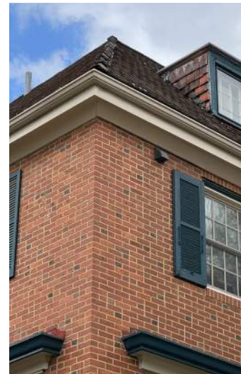
Example of a vent placed on secondary facade.
