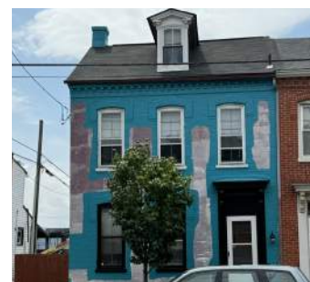
Example of inappropriate use of paint on masonry substrates, as well as inappropriate color choice.
