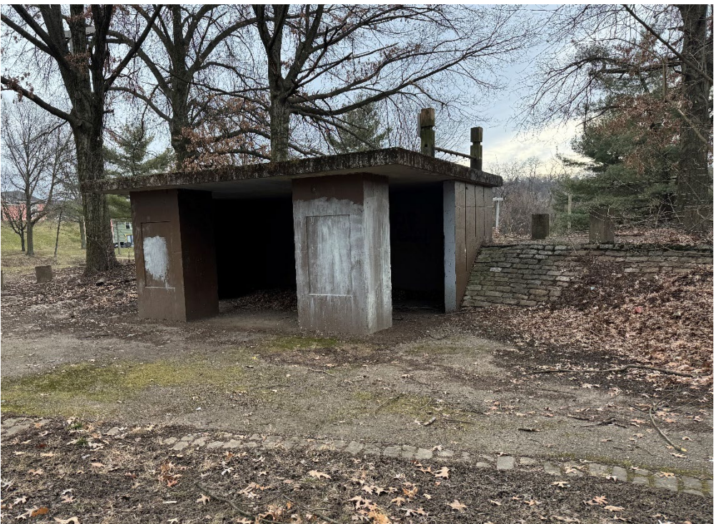
Address Structure at Former Play Area
